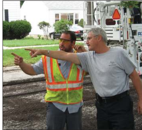
Public Works employee Steve Crowley and President Pulia discuss the details of the Public Works grinding project.
